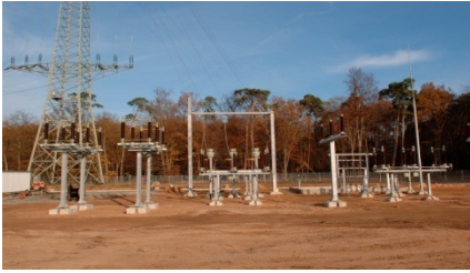
Power grid connection
