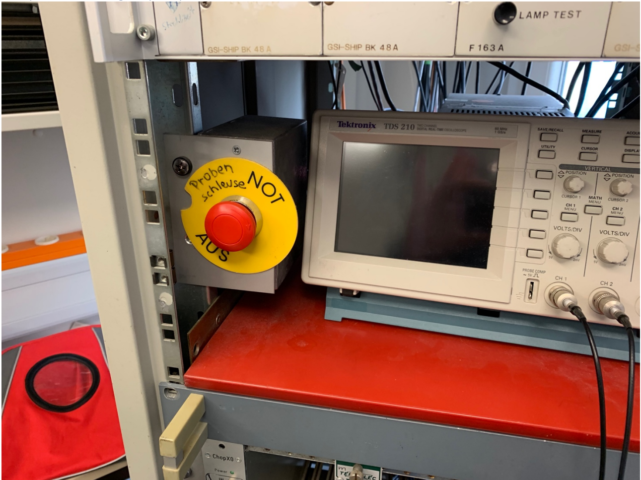
Figure 7 Emergency-stop for sample-inlet system
