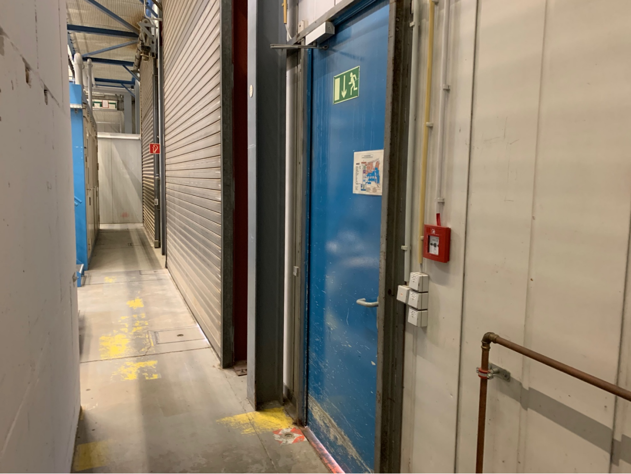
Figure 20 Emergency exit, fire alarm button
