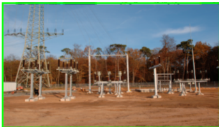
Power grid connection
