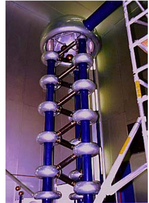
high voltage generator U = 400 \text{ kV}
